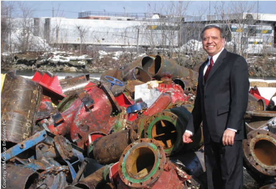
Pumping system design significantly affects district cooling system efficiency. Quite often, numerous pumps can be removed to save a facility energy and money. Hemant Mehta is shown here with 23 pumps that were removed from an 18,600-ton chilled-water system. Nine additional pumps were bypassed. The facility is reporting nearly $1 million in annual cost savings.
